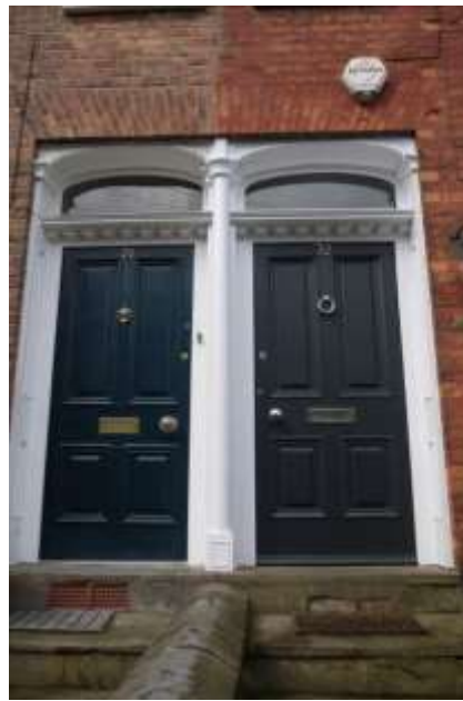
Original door on the left and a replacement on the right at Nos. 72-74 New Street
