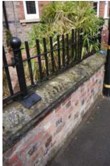
Reinstatement railings are generally poor quality and inappropriate
